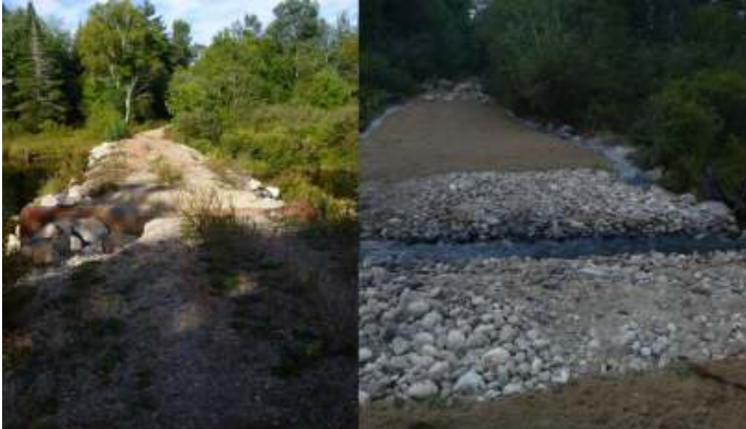
Figure 28. Beaverdam Stream culvert removal before and immediately after culvert removal and tree planting, 2015, Wesley, ME.
